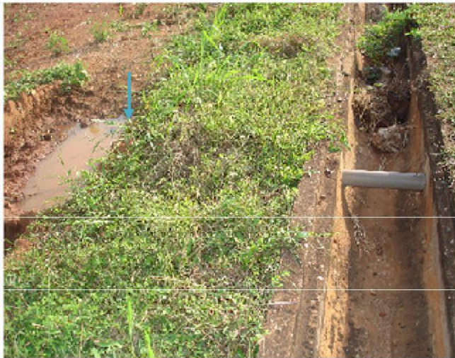
Figure 1. A broken pipe from construction work (Noguchi Memorial Institute for Medical Research, Legon, Accra, 2006). Arrow indicates direction of leakage on pipe.
