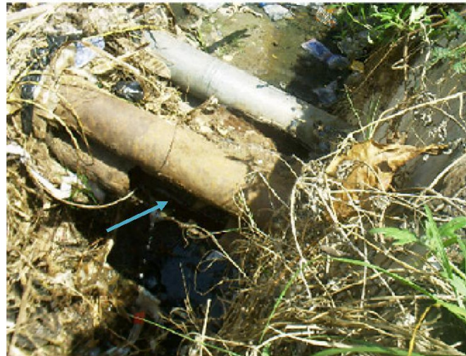
Figure 3. A broken metal distribution pipe (Danquah circle, Accra, 2006). Arrow indicates direction of leakage or breakage on pipe.
