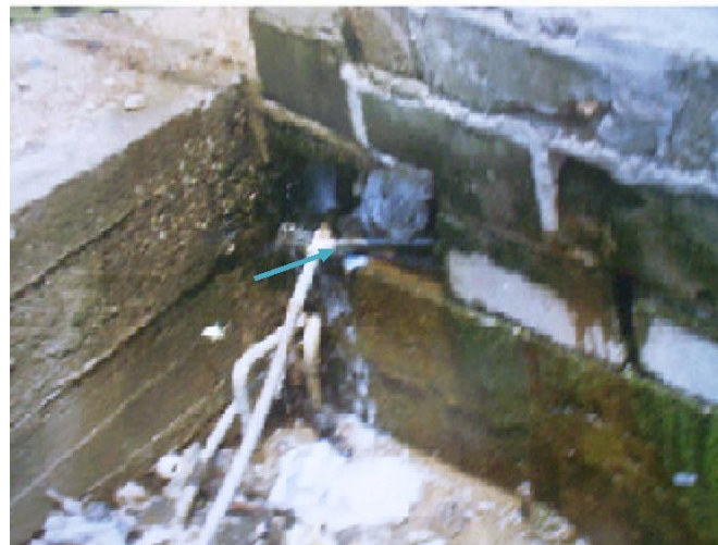
Figure 4. A broken pipe from improper sealing at a joint (New Fadama, Accra, 2006). Arrow indicates direction of leakage or breakage on pipe.
