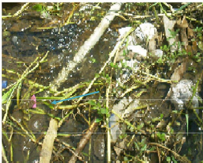
Figure 2. A broken pipe submerged in sewage water (Danquah circle, Accra, 2006). Arrow indicates direction of leakage or breakage on pipe.
